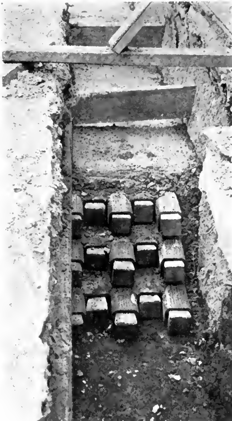
15 duct run showing concrete encasement.
